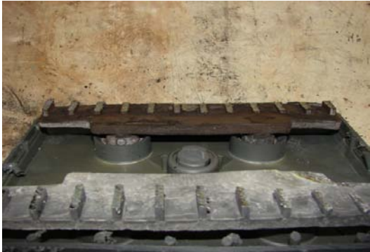
Figure 4. Examination of the internal lead hardware of the MP&L field-aged cells shows no signs of unusual corrosion or accelerated deterioration.
